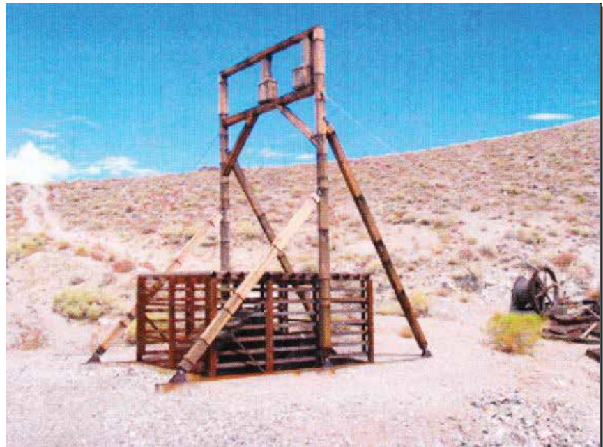
Cupola prevents people and animals from falling into an abandoned mine shaft. Photo courtesy of the California Department of Conservation.
